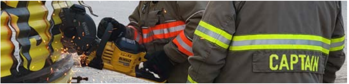
A first responder uses a circular saw to cut patterns into a grain bin square that will relieve pressure on the grain bin wall and prevent it from toppling over to one side. The openings also provide access to the grain bin so rescue procedures can be carried out. All photos by M. Charles Gould, Michigan State University Extension.
